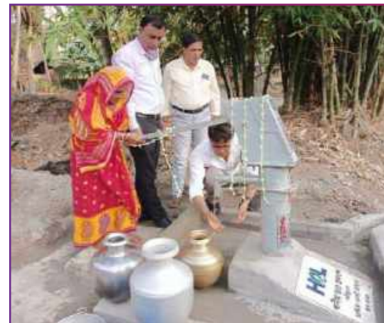
Installation of bore well for safe drinking water for nearby Jhikurkhali village
