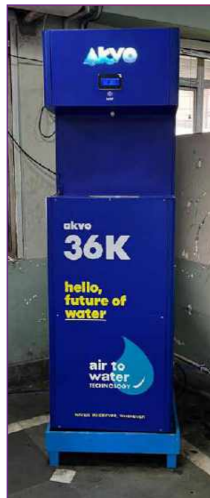
Air to Water Generator at BBGS
